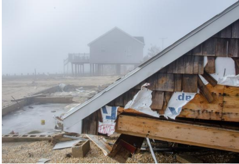
Ocean Gate, N.J., Jan. 30, 2013 -- The home on pilings, in the background, survived Hurricane Sandy with relatively little damage, while its neighbor (foreground) was not as fortunate. Photo by Liz Roll/FEMA
